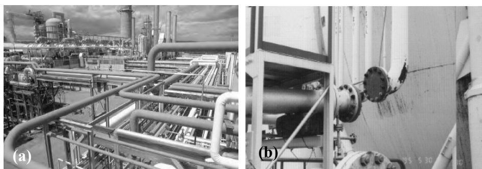
Fig. 6. (a) A piping system in a refinery, (b) Breakage of a piping flanged connection.
