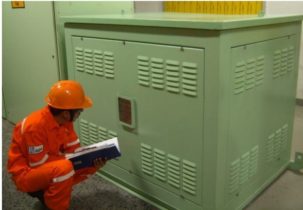
Fig. 3.6.2. High resistance transformer installed in a petrochemical plant.
