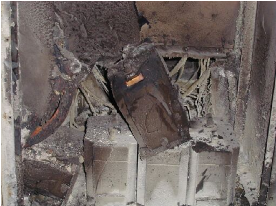
Fig. 4.3.1. Damage to the PT and panel where PT was connected.
